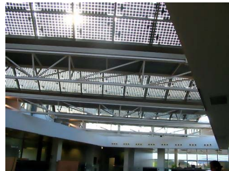
Fig. 7 Isofóton, Spain. Detail of the monocrystalline cell modules [10]
