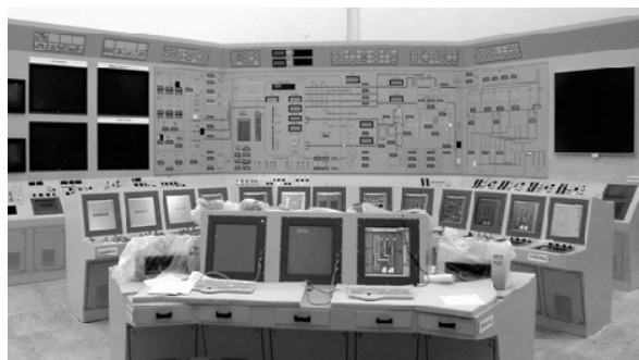
Fig. 1 Modern Main Control Room of the NPPs
