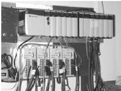
Fig. 2 A large PLC
