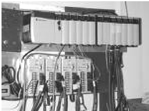
Fig. 2 A large PLC
