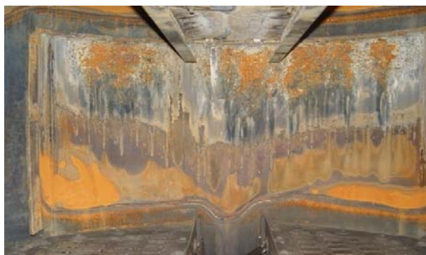
Fig. 1 Corrosion on shell on vapor area
