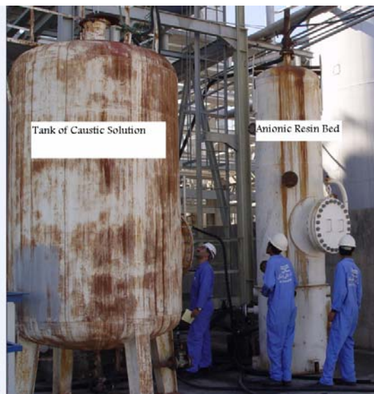
Fig.7 DEA Package recovery (left vessel Caustic Solution tank , right Anionic Resin Bed)
