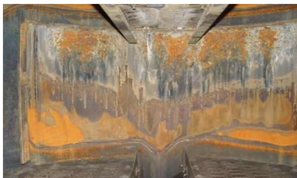
Fig. 1 Corrosion on shell on vapor area
