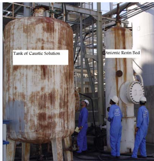
Fig.7 DEA Package recovery (left vessel Caustic Solution tank , right Anionic Resin Bed)
