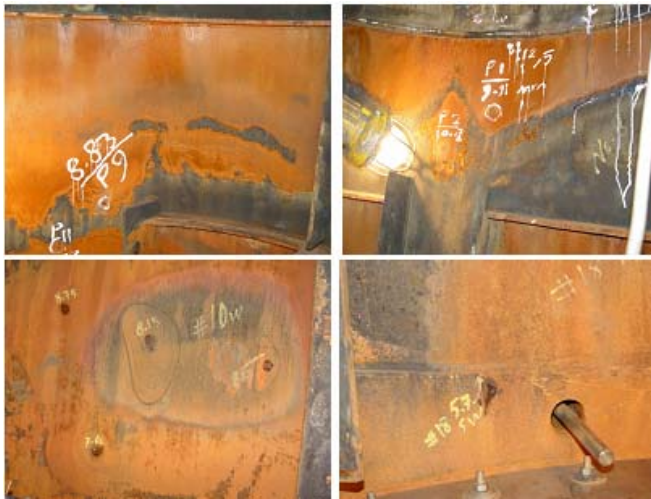
Fig. 3 CORROSION on Different Side of Shell(Top left to right ,Tray 9,Tray 8,Bottom left to right ,Tray 10,Tray 18)
