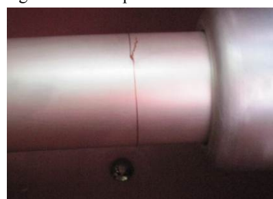
(a) Tip on the high-voltage conductive pole
