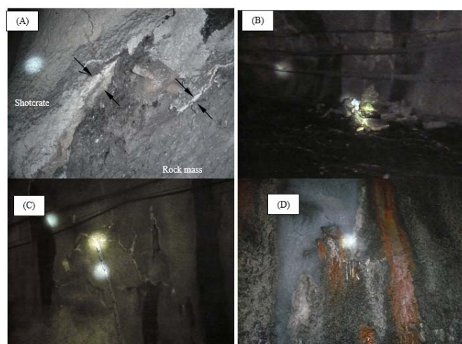
Fig. 1 Found problems in the shotcrete: (A) poor thickness, (B) detached blocks, (C) cracking, (D) leaks and oxidation
