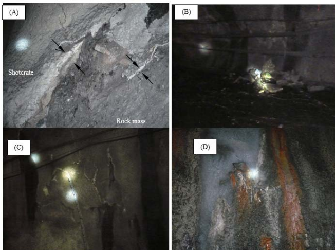
Fig. 1 Found problems in the shotcrete: (A) poor thickness, (B) detached blocks, (C) cracking, (D) leaks and oxidation
