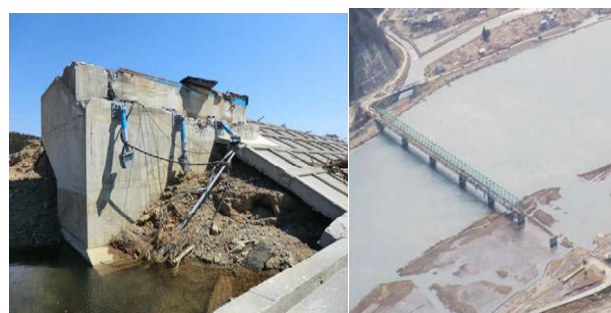
Fig. 2 Washed away girder bridge and truss bridge
