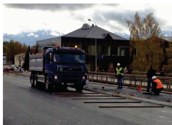
Fig. 2 Vehicle driving over planks paced on the road surface
