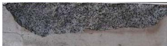
Fig. 4 State after testing – spalled concrete
