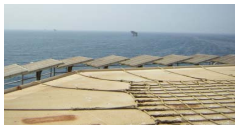
Fig. 2 Solar panel on unmanned platform
