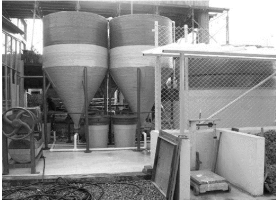
Fig. 1 Raw wastewater treatment plant
