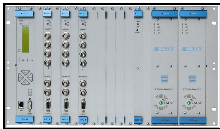
Fig. 1 None contact probe connection main board in substation
