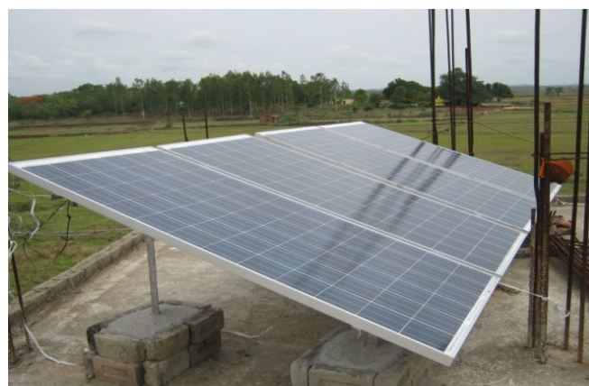
Fig. 8 Rooftop PV system
