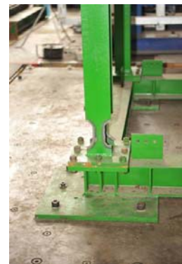
Fig. 2 Flange partially cut-out at the bottom end of column
