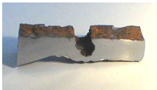
Fig. 1 Severe preferential weld corrosion in carbon steel pipeline carrying inhibited oil and gas [8]
