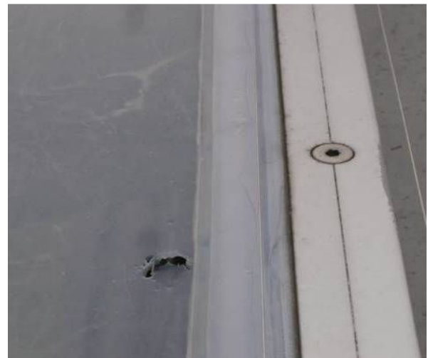
Fig. 16 Picture of Hanover stadium roof – holes close to an edge
