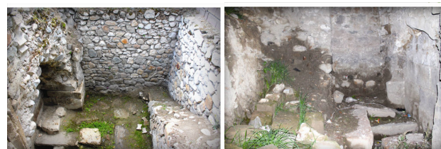
Fig. 10 Fountain deteriorations (material losses, vegetation on the sides, dampness, mossiness problems from the ground etc.)
