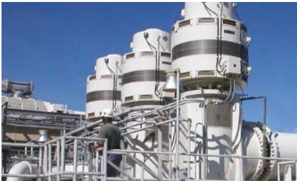
Fig. 1 Typical sea water vertical Centrifugal lift Pumps
