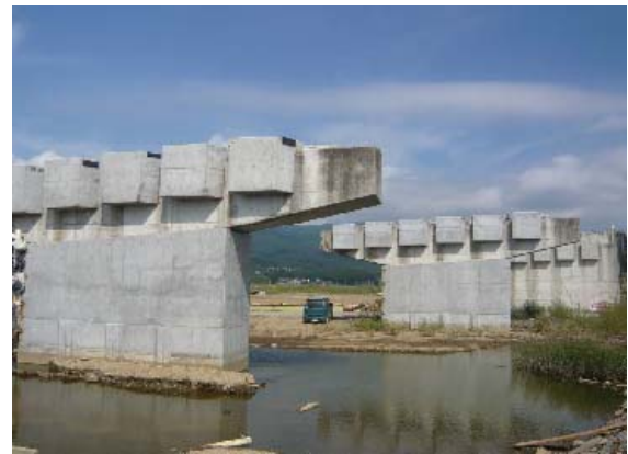
Fig. 5 Damaged Numata-Kosen bridge during Tohoku Tsunami
