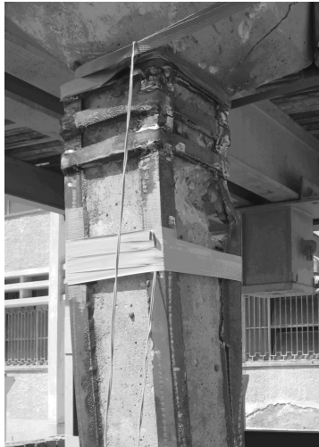
Fig. 6 Failure of columns strengthened with unequally distributed straps
