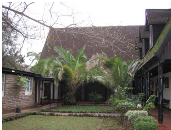
Fig. 11. Main Building at the Nairobi Zoo, Kenya. The use of 'cavaco' for the roofing. A technology extensively used by the Ribeirinhos and the indigenous people in the Amazon region.
