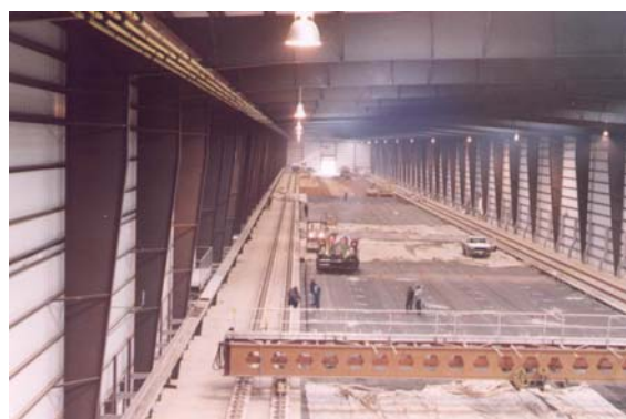
Fig. 1 Inside view of NAPTF during construction of test pavements (Photo Courtesy: NAPTF)
