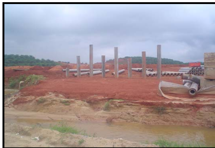
Fig. 1 Construction of integral bridge at Phase 2 of East Coast Expressway, Malaysia (Akib, 2009)
