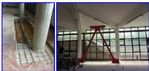
Fig. 17 Construction of the additional R/C beam in one of the two DB alignments parallel to x in the pilotis wing
