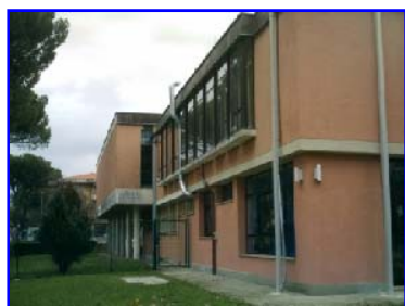
Fig. 10 Views of the building before the seismic retrofit and architectural renovation interventions
