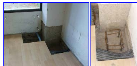
Fig. 16 Preparation of the anchorage zones of braces to the foot of a column
