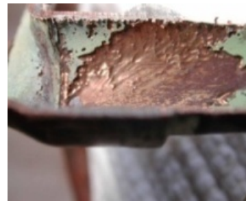
Fig. 10 Copper pipe corrosion
