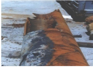
Fig. 1 Ductile iron pipe failure
