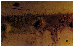
Fig. 2 Ductile iron pipe corrosion
