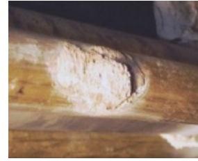
Fig. 6 Galvanic ringworm corrosion
