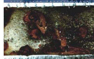
Fig. 7 Corrosion of galvanized potable water piping
