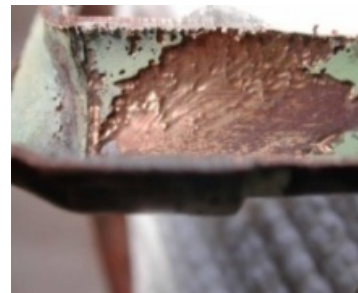
Fig. 10 Copper pipe corrosion
