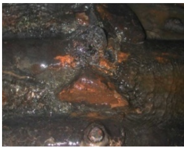
Fig. 14 Culvert pipe corrosion
