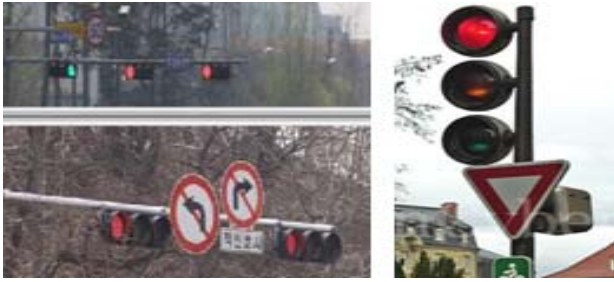
Fig. 1 Left picture is horizontal traffic lights and right picture is vertical traffic lights
