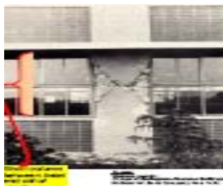
Fig.4. large window openings AND SHORT COLUMN
