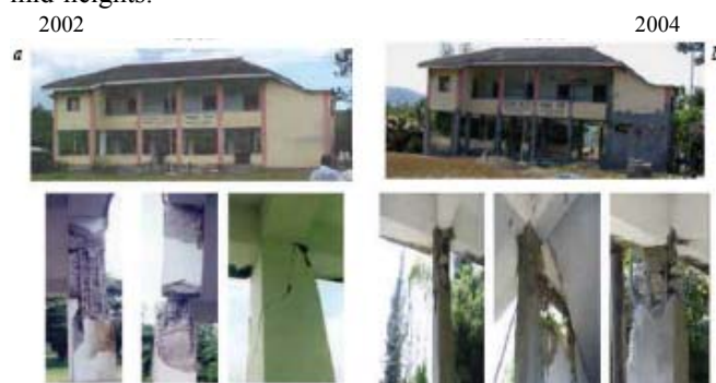
Fig. 10.a.Severe Cracking and Damage to soft first storey columns of Nabagram Panchayat Bhavan building primarily due to 'missing' ties in 2002 earthquake, b.more damage in 2004 earthquake to same columns which were 'retrofitted'[9].
