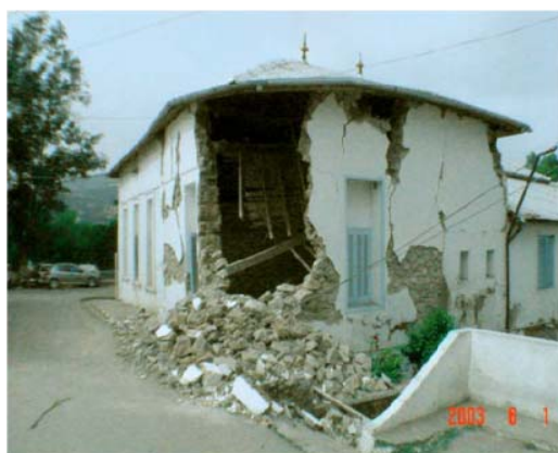
Fig. 8 Partial collapse of walls due to the 2003 Boumerdes earthquake
