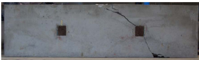
Fig. 11 Crack pattern for beam S05-80-3 [12]
