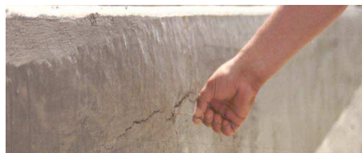
Fig. 2 Crack in Barrier
