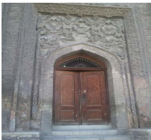
Fig. 4 Moisture along with fluctuations in temperature can lead to disintegration of the façade (plasterwork) in cold regions (Alavian dome, Hamadan, Iran)
