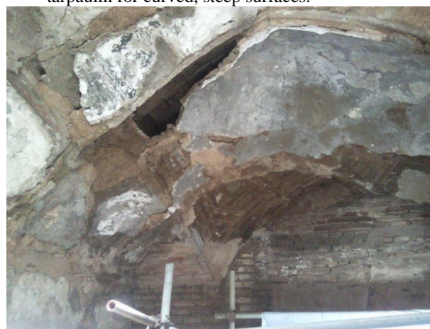
Fig. 7 Damages due to descending moisture (Vakil Bath, Shiraz, Iran)
