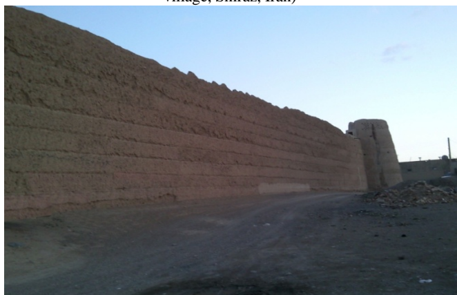
Fig. 2 destruction and erosion of an earthen building due to climatic factors (Damab castle, Isfahan, Iran)
