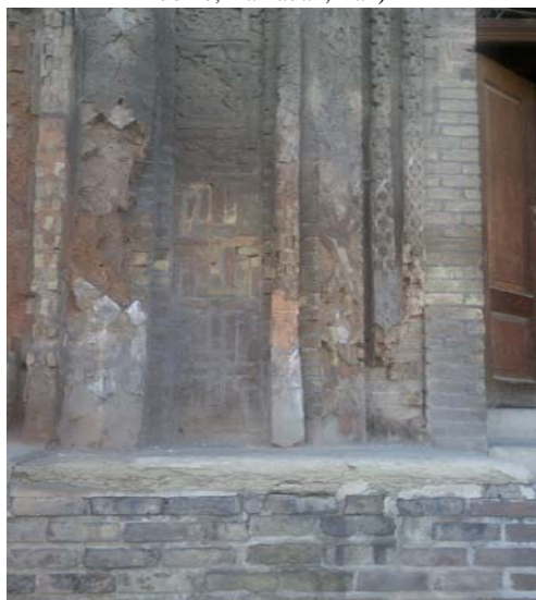
Fig. 5 penetration of moisture into the pores of the building and freezing between the bricks which shatters them in cold regions (Alavian dome, Hamadan, Iran)
