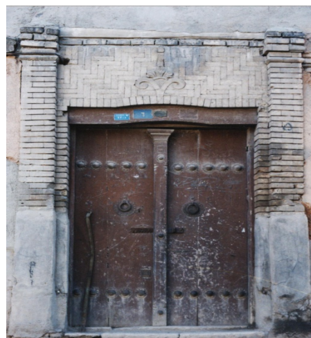
Fig. 6 Damages due to ascending moisture (Jewish Synagogue, Hamadan, Iran)
