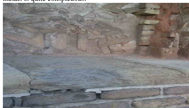
Fig. 3 Decomposition of stones due to acid rains
