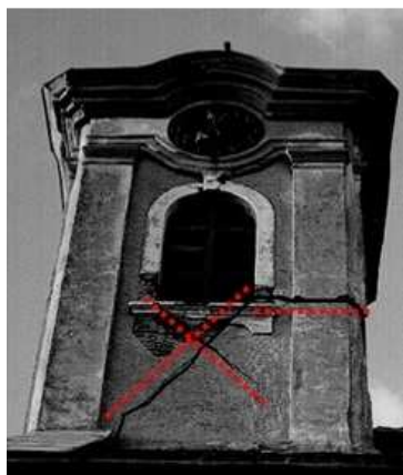
Fig. 15 Cracks at bell tower
