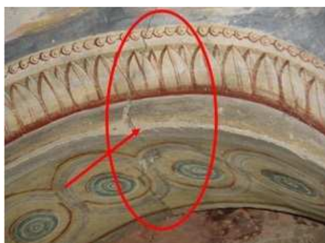
Fig. 16 Cracks at arches
