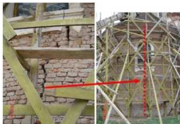
Fig. 14 Cracks at the eastern wall
