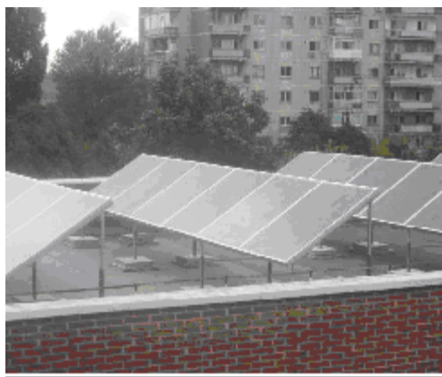
Fig. 5 PV plant on the Polytechnic University Bucharest
