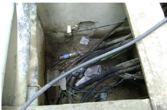
Fig. 14 Electric cable trench was found uncovered
