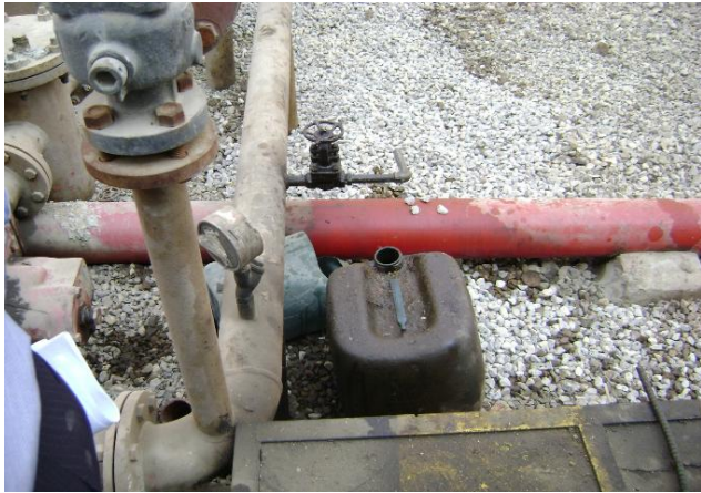
Fig. 10 Housekeeping of tank zone was found poor
