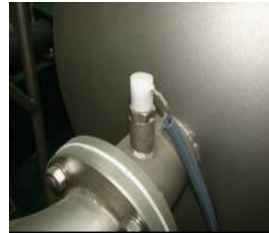
Fig. 9 PT100 Temperature sensor
