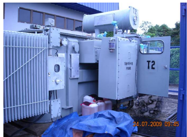
Fig. 1: Transformer under study
