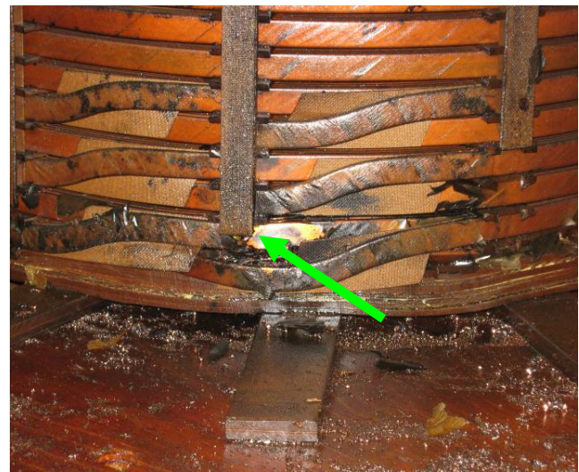
Fig. 12: Arrow shows the arcing spot
