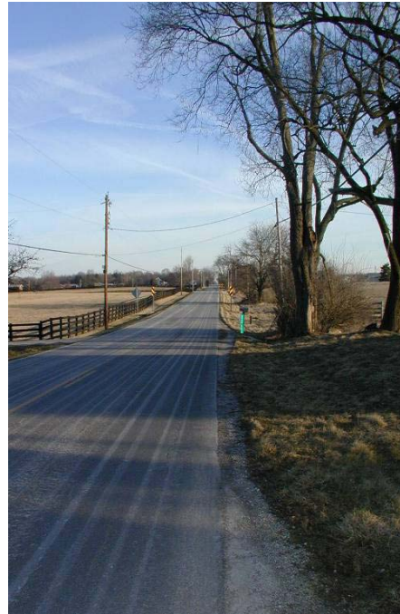
Fig.1 Failing Delaware County Pavement
