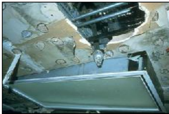
Fig. 2 Piping Failures in 1994 Northridge Earthquake (Miranda, 2004)
