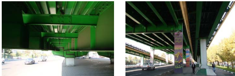
Fig. 3 Left Photo: South view of Gisha bridge, Right Photo: North view of Gisha bridge
