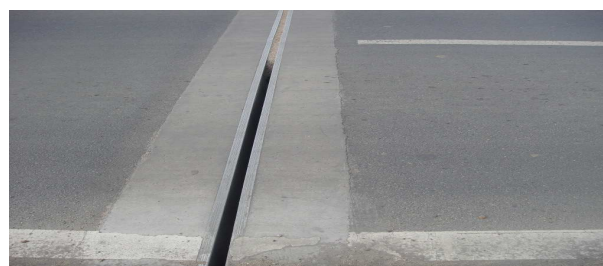
Fig. 4 (b) Losing of joint material
