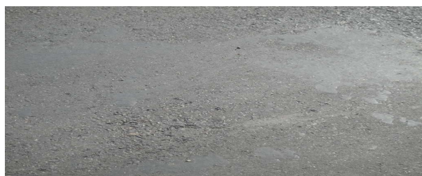
Fig. 5 (b) ) Bleeding of asphalt
