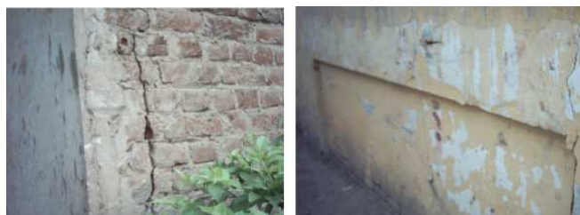
Fig. 2 Longitudinal cracking occurs in buildings
