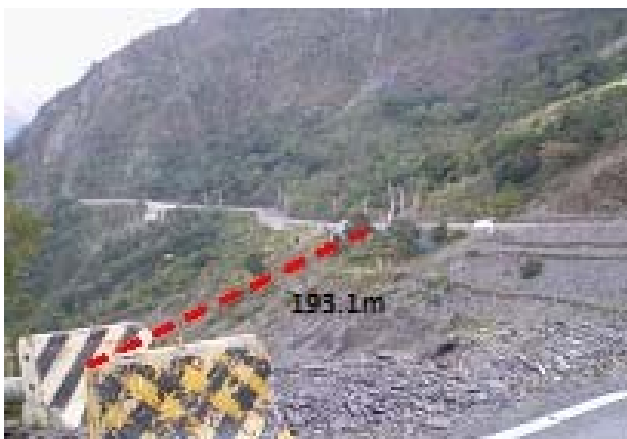
Fig. 1 Location of slope collapse and sliding
