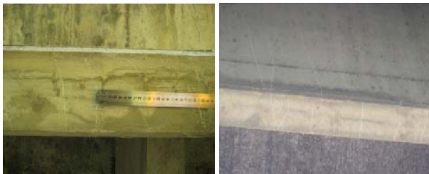
Fig. 9 (c) T beam cross-cracks in the region
