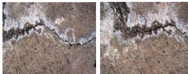
Fig. 6 South side of the pier # 5 surface cracks whitening
