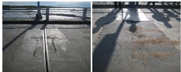
Fig. 11 Serious damaged bridge deck expansion joint
