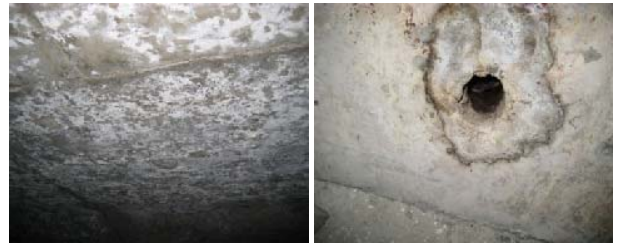
Fig. 9 (a) the internal box water drainage damage
