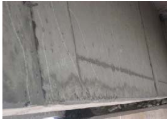
Fig. 9 (b) T beam cross-cracks in the region
