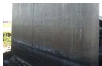
Fig. 7 Transverse cracks Pier #11
