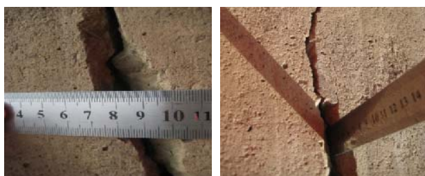
Fig. 5 5 Pier # 5 crack depth
