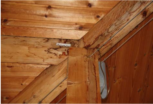
Fig. 1 Convective moisture ingress through a leakage at the connection point of bay and timber frame
