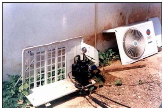
Fig. 3 Photograph of condensing unit of M-AC
